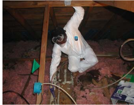
Air leaks are sealed at the attic floor to prevent conditioned air from escaping the living space
